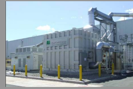
1.4 MW power plant
