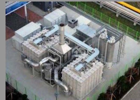
2.8 MW power plant
